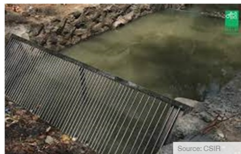
Poorly designed Screen on open drain
