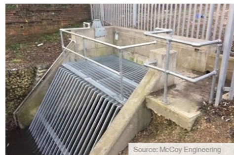
Screen on open drain with raking platform
